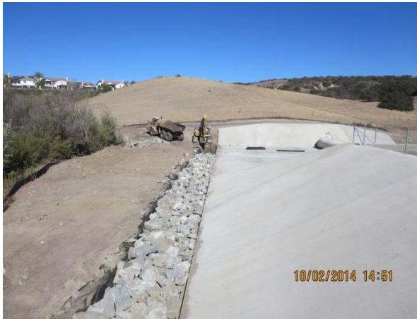
Rip upstream of lower dam
